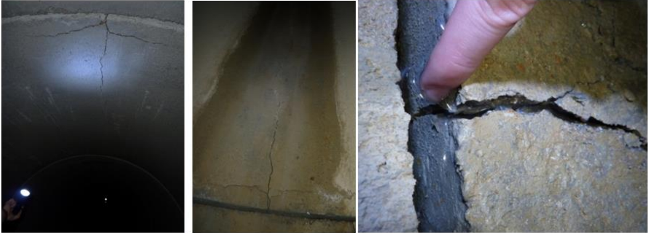
Figure 2. Observed damage. Source: Own elaboration (2017).
